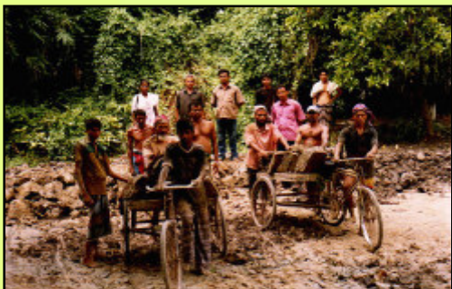
Soil is carried by tricycle to raise ground level to build a flood shelter.
