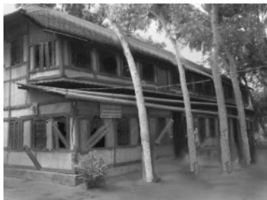
Old Multipurpose Mission Center severely damaged, deemed unfit for use
